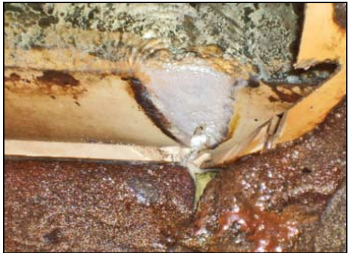
Running infiltration from invert & bench interface.
